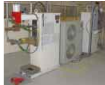
Water Recirculating Equipment
