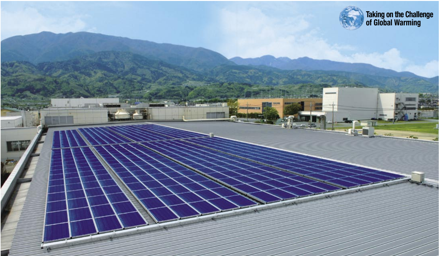
Our photovoltaic power generation system in use at TDK Corporation's Kofu Plant
