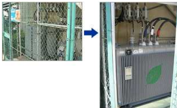
Before: 257,653 kWh → After: 228,530 kWh Power loss reduced by 11.4%
