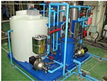
Equipment for processing wastewater for reuse
