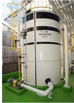
Recycled water storage tank.
