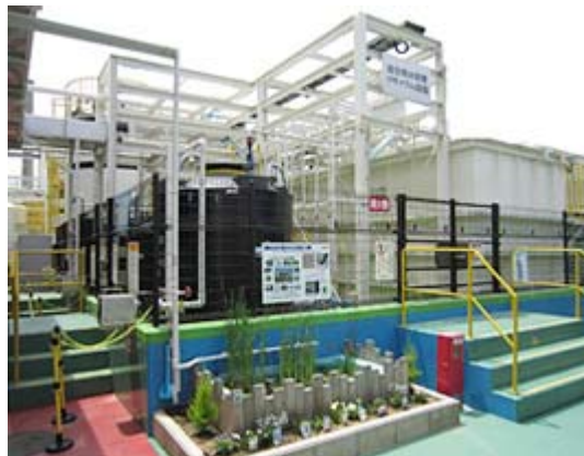
Water recycling equipment for new metal plating process
