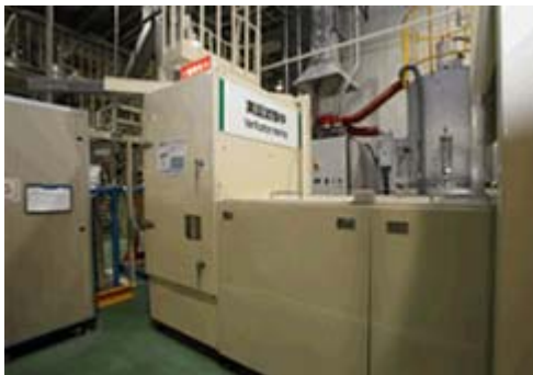
Equipment for removing plastic containing bromine (Equipment for X-ray analysis separation: undergoing testing)
