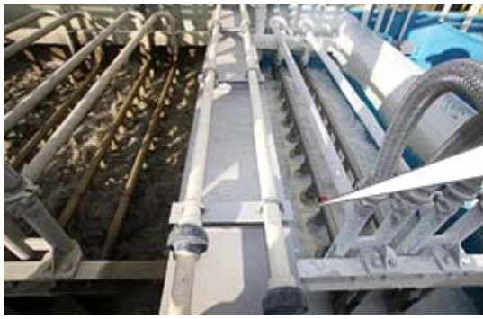
Water detoxification equipment at metal plating facility. Vat at left is for heavy metals; vat at right holds water containing fluorine.
