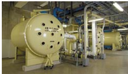
Ozone generation equipment
