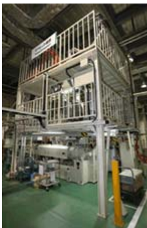
Pelletization equipment (Equipment for creating pellets of recycled high-purity plastic)
