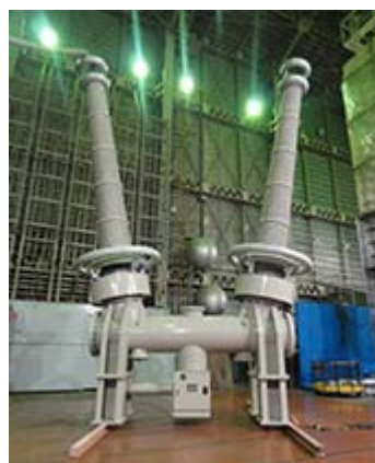
Gas circuit breaker
