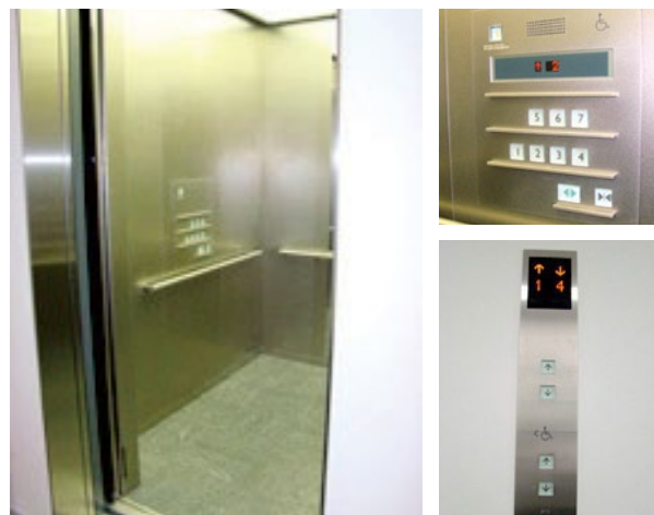
Barrier-free elevator (Advanced Technology R&D Center)
