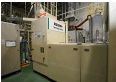
X-ray sorting equipment for removing plastics containing bromine
