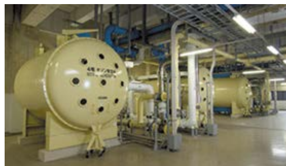
Ozone generator delivered
