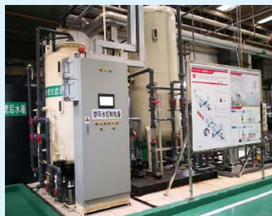
Water recycling facility
