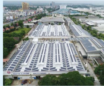
Solar power generation system utilizing roofs
